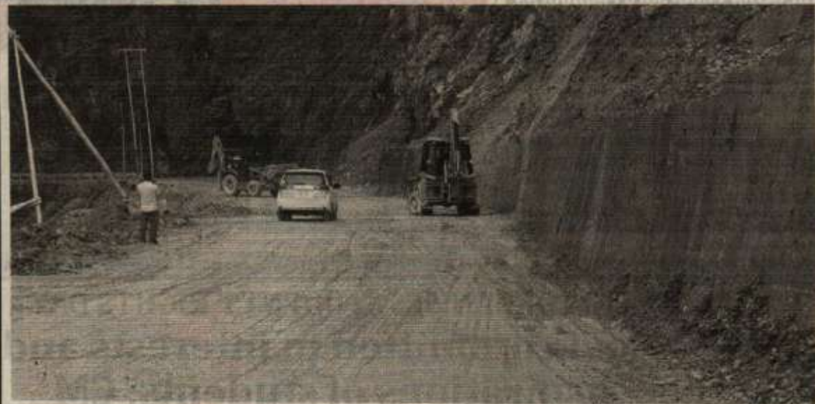
SETI JHORA CLEARED, FOR NOW: Finally, after five days of uncertainty two-way traffic was restored at Seti Jhora on Sunday afternoon. A break in the rain and the courage and diligence of West Bengal PWD's JCB pilots helped clear the debris enough for vehicles to get unimpeded travel through the area.
