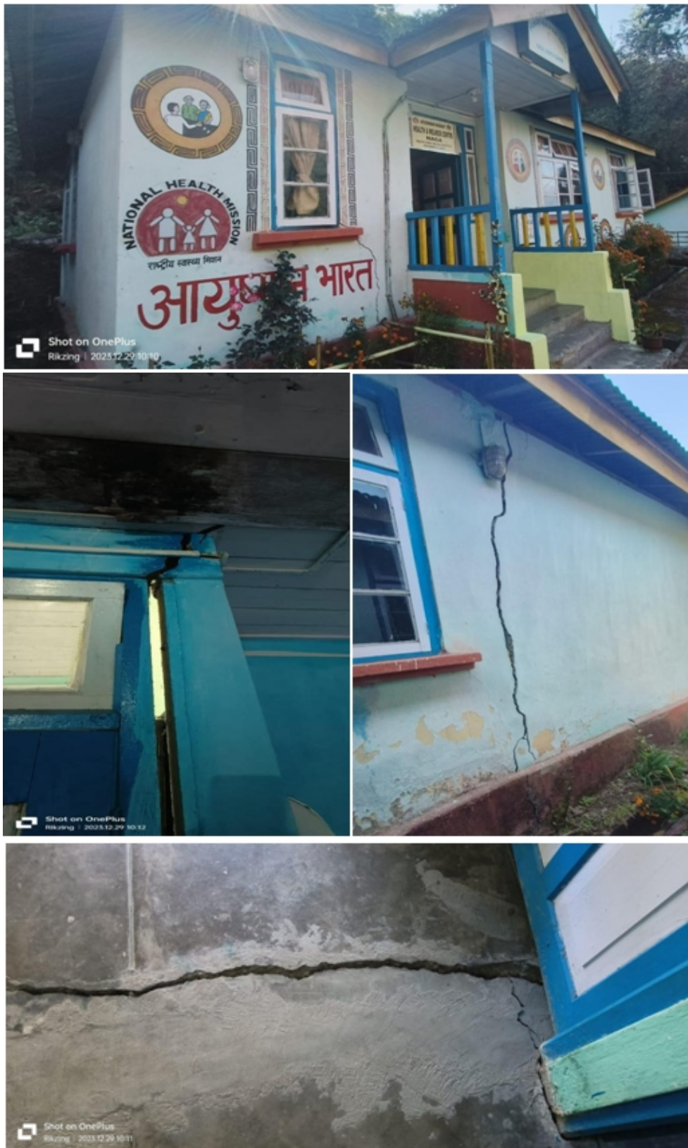
Figure 1 Damages to Naga Health and Wellness Sub Centre
