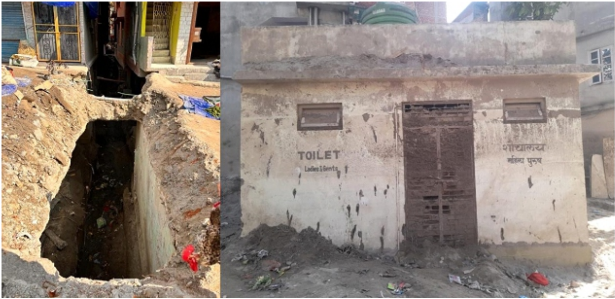
Fig: damaged drain singtam- toilet -Ramgpo
