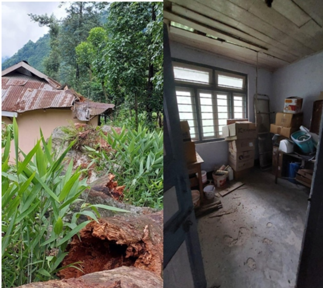
Figure 2 Damages at Makha Health and Wellness Sub Centre, District Gangtok
